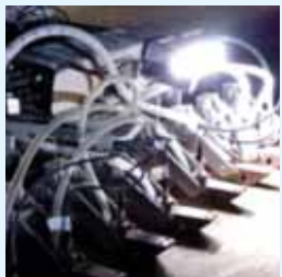
Decatur, US mapped out their coal boiler water tube thickness to detect wear spots
